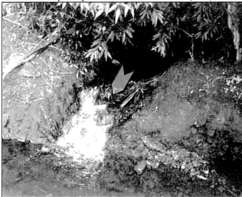
Photo 2. Honopou Siphon Intake at Lowrie Ditch (L-16).
